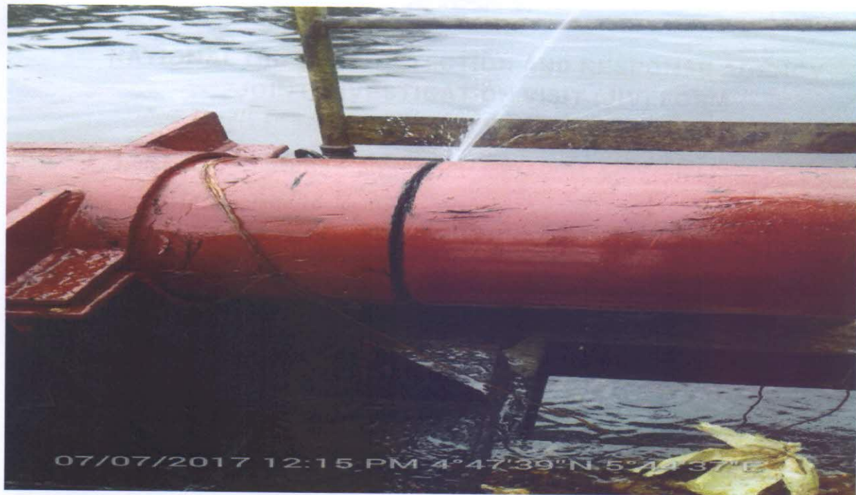
LEAK POINT- HACK SAW CUT OF ABOUT 150MM
